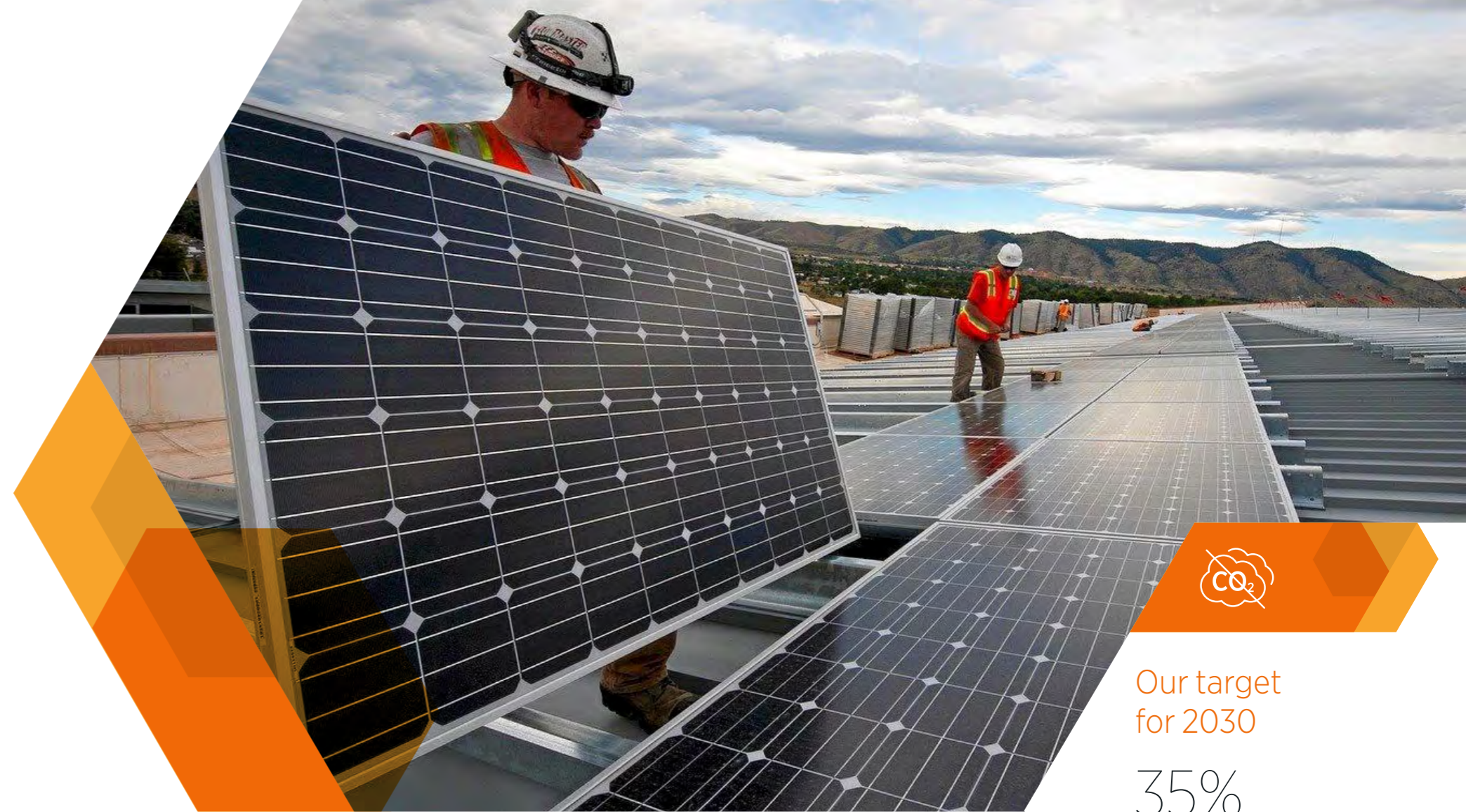
Photovoltaic installation in Colombia
