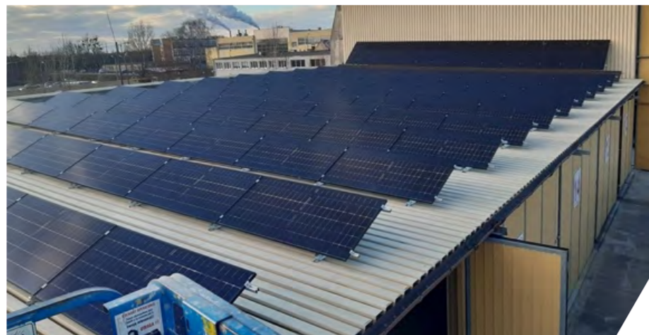
Photovoltaic installation at Etex Konin (Poland)
